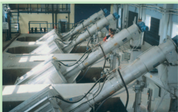
Stainless steel rotary drum fine screens with integrated screenings washing installed in parallel (Photo: HUBER SE, Berching, Germany)
