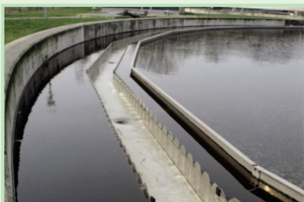
Stainless steel overflow gutter (Photo: Informationstelle Edelstahl Rostfrei, Düsseldorf, Germany)
